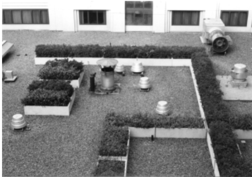
Figure 8-4. Part of the investigation process should include inspection of the exhaust vents and air intakes to ensure they are not located too close together, resulting in the building feeding bad air back into itself.
